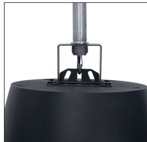
Pipe with safety cable
